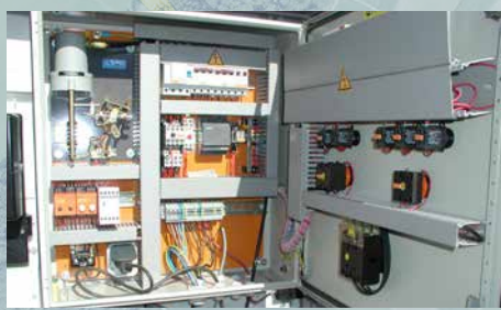
Station de pompage Dielchen
